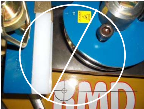
Too far away from die
